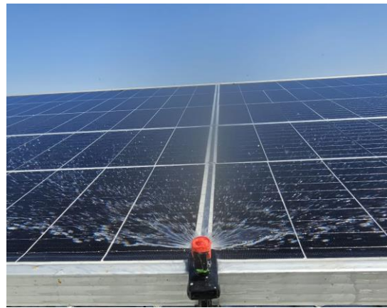
For Solar Panels washing
